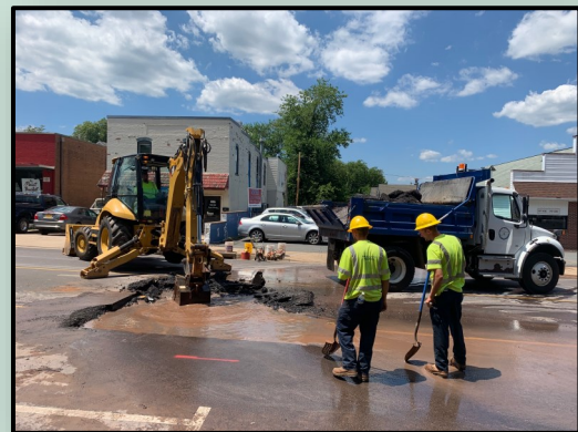
Main Street Water Main Break & Repair
